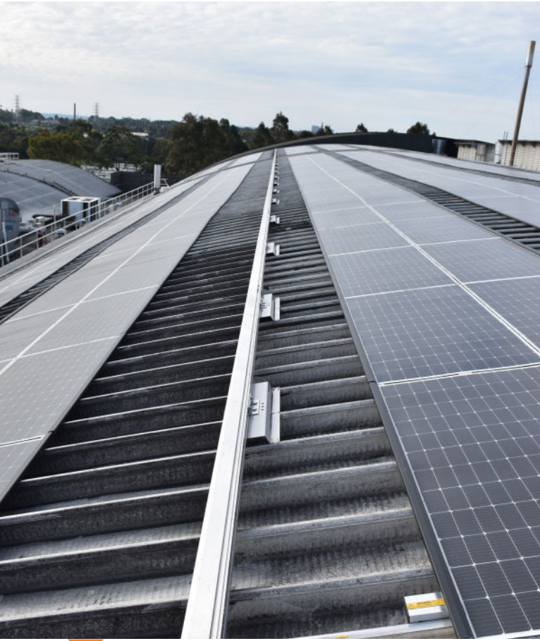
Rigid rail system to allow for installation and maintenance of the solar panels.
