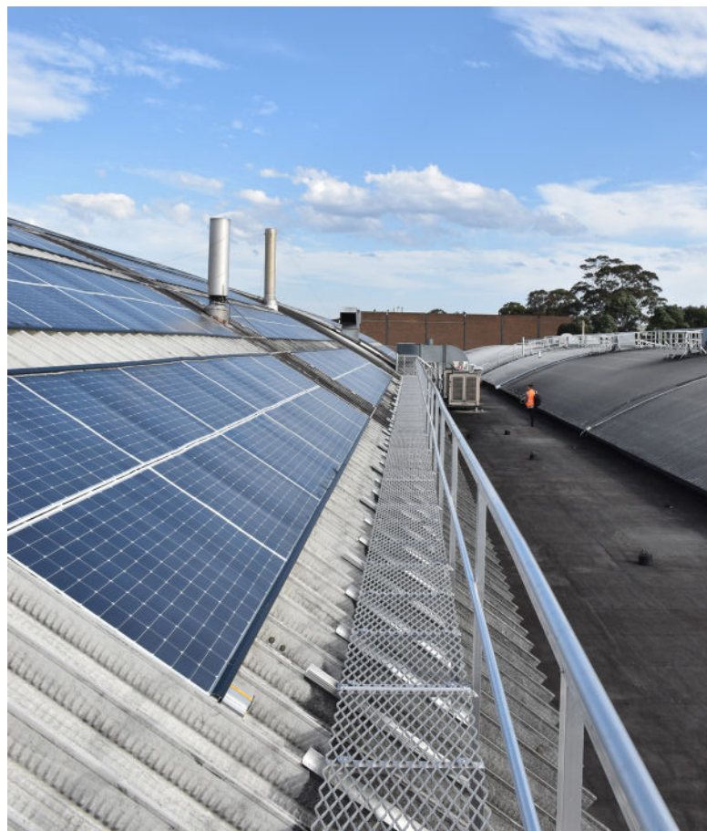
Levelled walkway installed at the base of the roof for servicing the solar panels.
