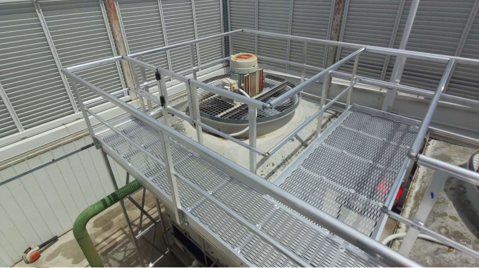
Free standing cooling tower platform with guardrail and self-closing gate.
