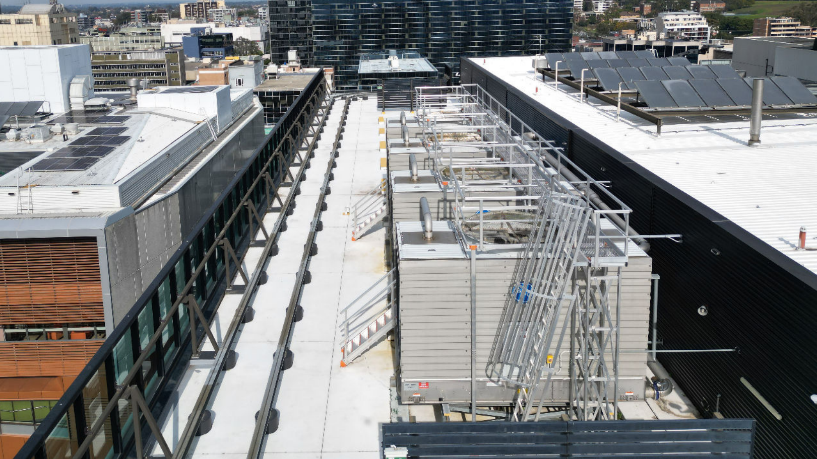
Elevated platform with guardrail both sides and angled cage ladder to access the platform.
