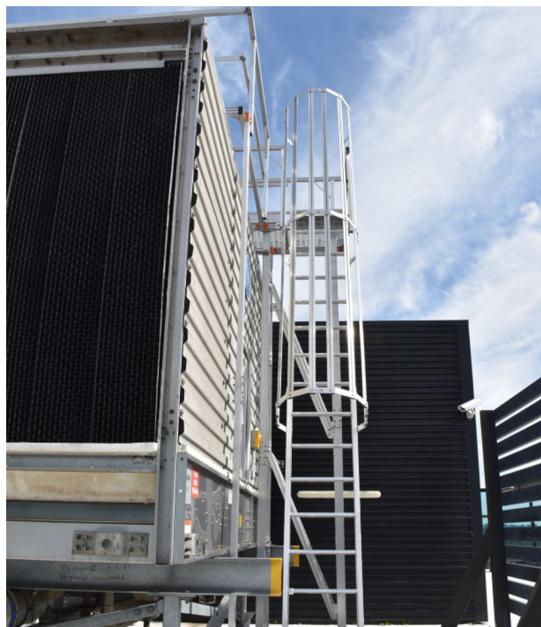
Angled cage ladder system integrated with platform and guardrail system.
