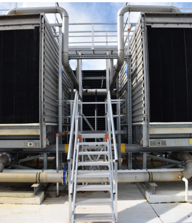
Stair & platform system installed for safe access to lower areas of the cooling towers.
