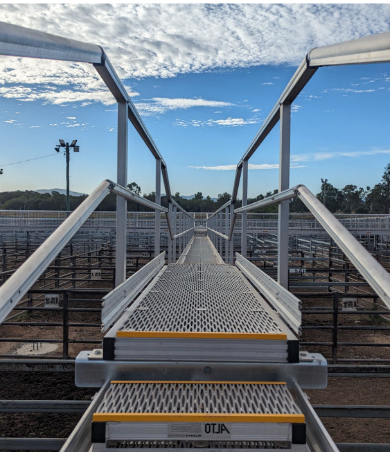
Raised step bridge system to accommodate plant and equipment passing through the yards.
