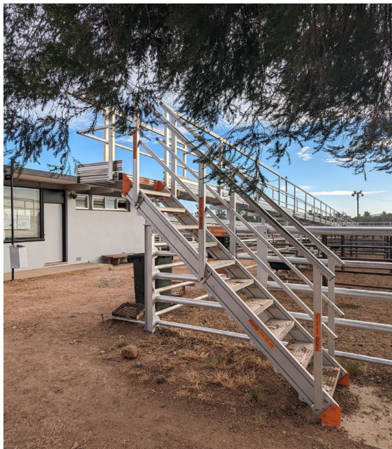
One of the 21 stairways to allow safe access onto the various areas of the auctioneer platforms.
