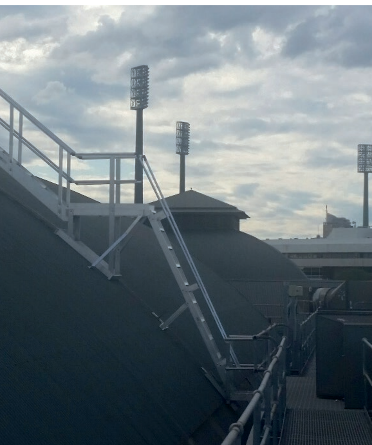
Step Ladder from lower plant platform to midway platform.
