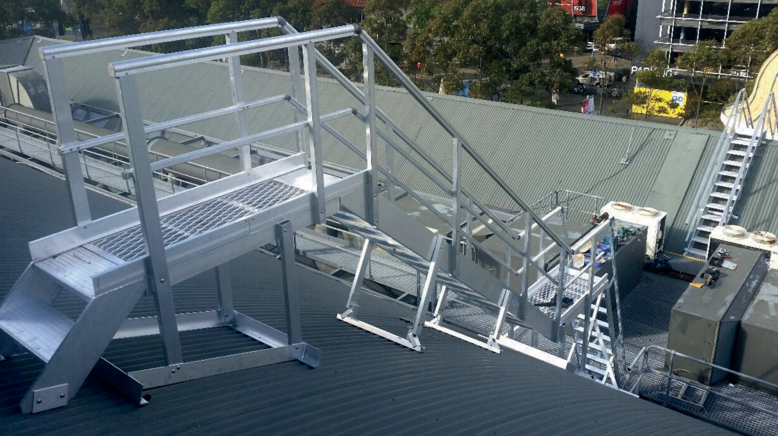
Step Ladder and stair system to traverse the curved roof.
