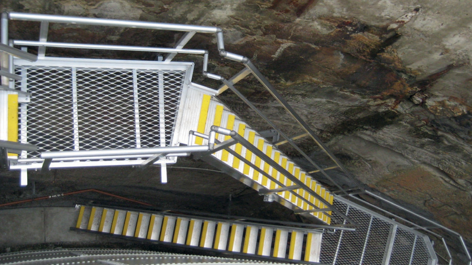
Design & construction of aluminium stairs for access down 13 metre cliff into a confined space area.
