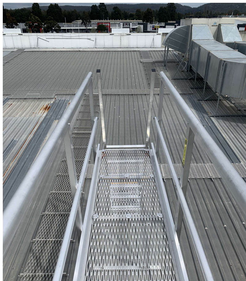
Landing platform ensuring ease of access on the roof
