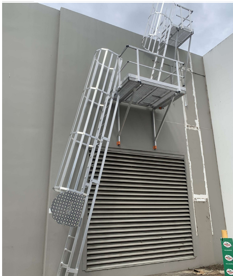
Angled caged ladder with landing platform & lockable gate
