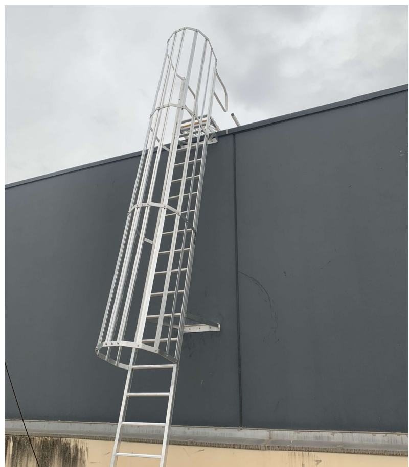
Caged Parapet step ladder system
